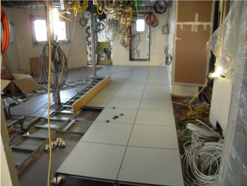
Data floor in Ops center
